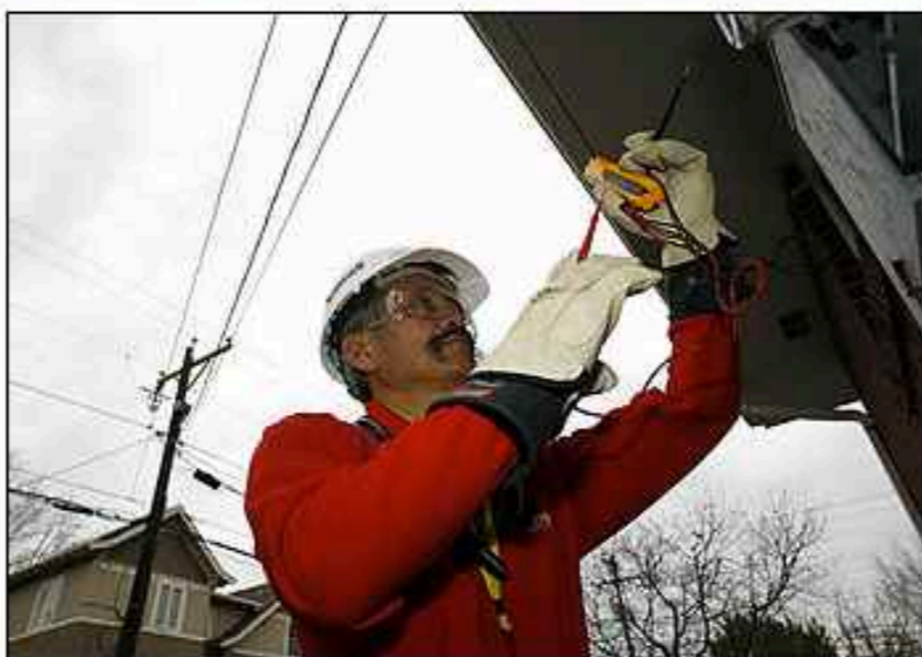
Electric utilities receiving "smart grid" grants must ensure cybersecurity. (By David Zalubowski - Associated Press)
